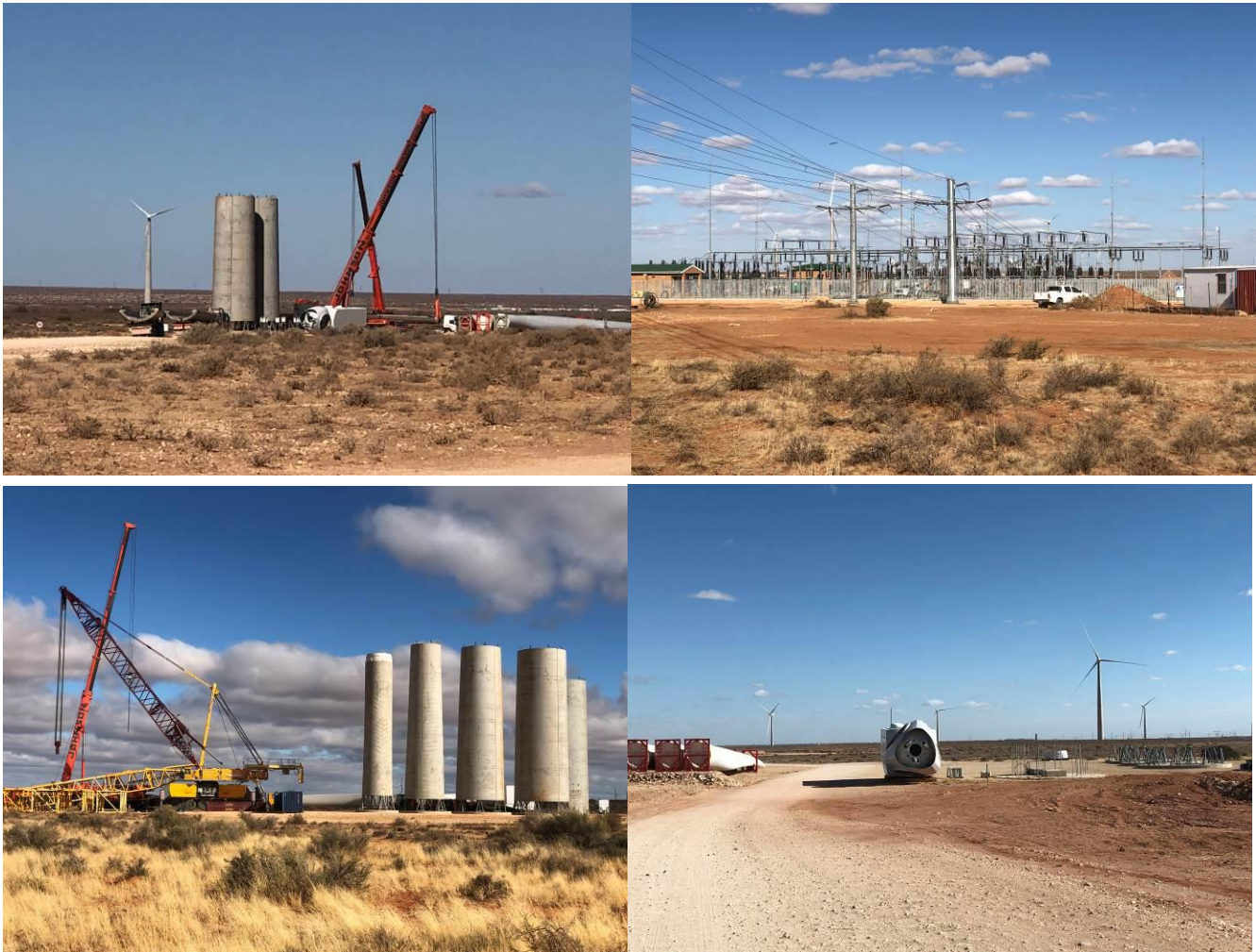
Figure 2-3: Photographs depicting the construction phase of a wind farm similar to Botterblom WEF.
