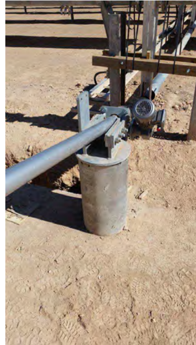
Figure 36: Motors used in the single axis tracking system should be AC brushless.
