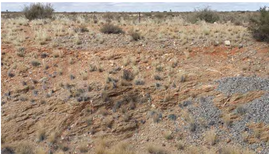
Figure 11.7: Photograph from the area of typical soil profile in a railway cutting showing shallow bed rock (Mispah soil form).
