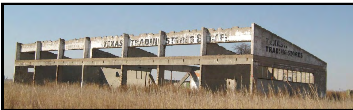
Figure 17: Dilapidated structure (number 5 in Figure 13)
