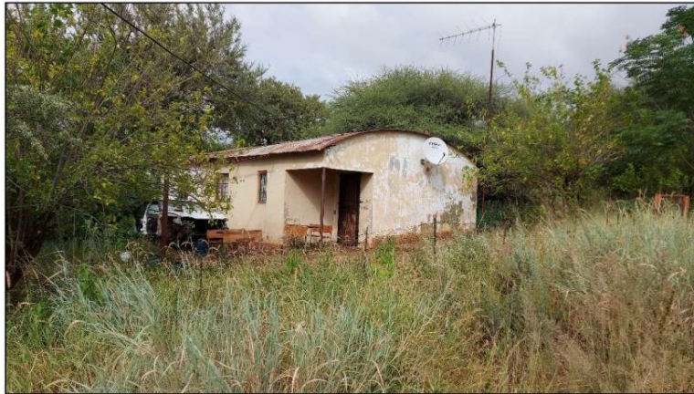
Figure 34: Another remaining building at Site B03.
