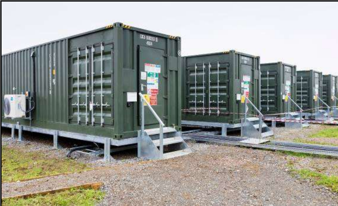
Photograph 1.2: Example of BESS located in storage containers
