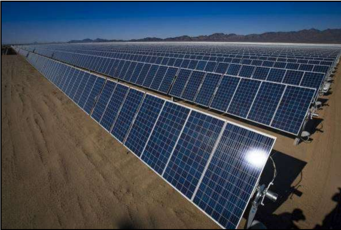
Photograph 1.1: Typical PV SEF facility
