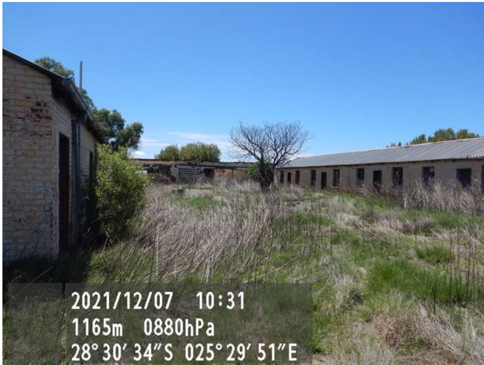
Figure 16: Gutters that needs to be maintained.
