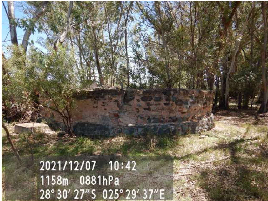
Figure 14: Old dam that is filled with building rubble
