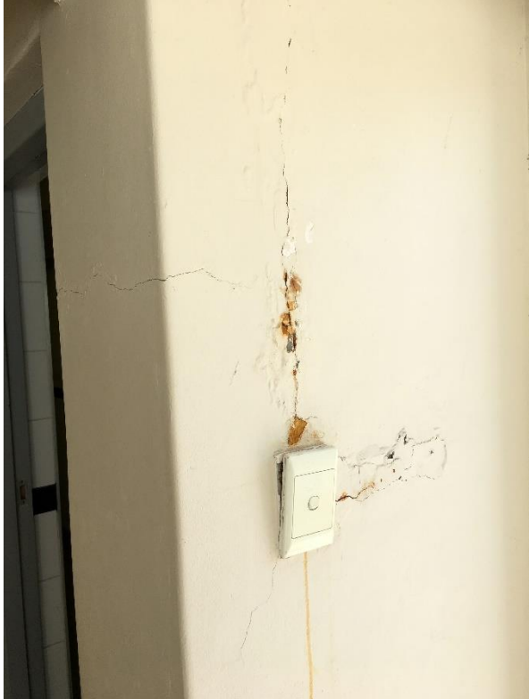
Conduiting to be replaced and switch made good
