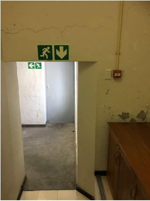
Surface mounted conduit to be recessed
