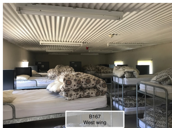
Fig 6. Note the flaking paint on the walls close to the concrete ceiling. Most likely caused by excessive moisture generated by children with walls not being able to 'breathe'.
