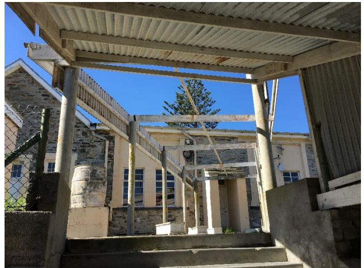
Lighting required along stairway
