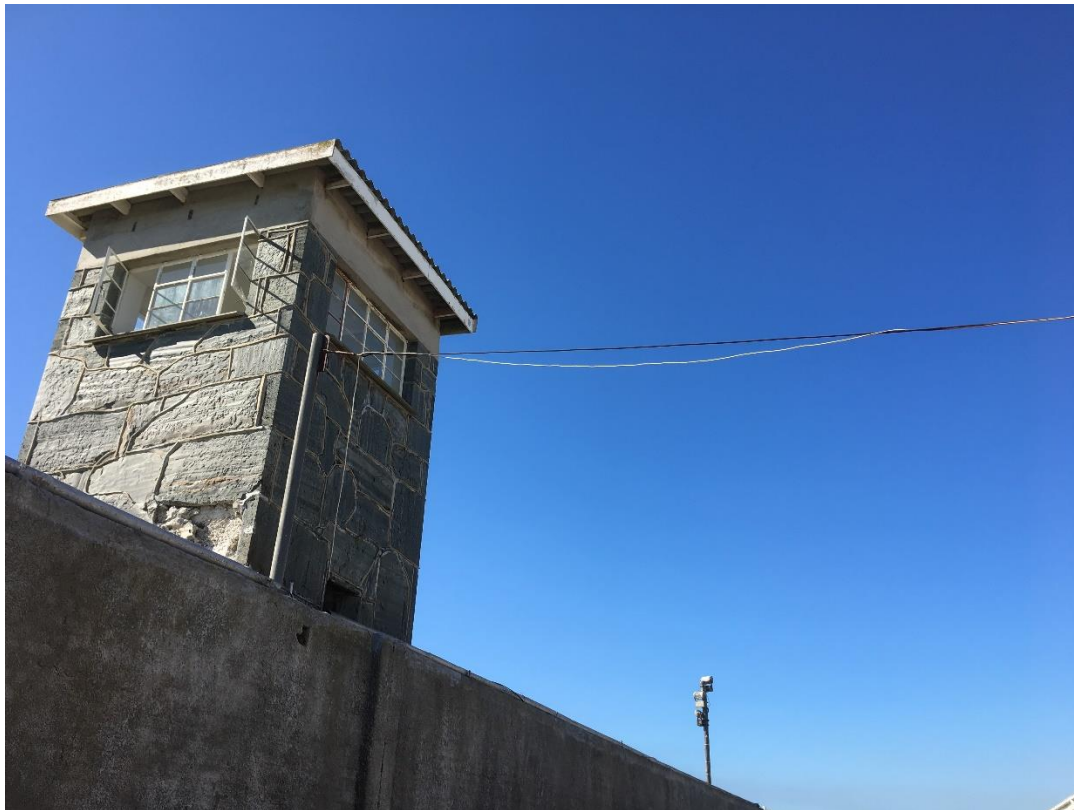
Remove loose overhead cable/extension between Main Kitchen & watch tower
