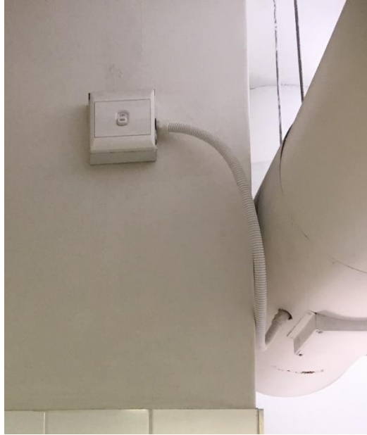
Electrical supply to be corrected and Isolator recessed
