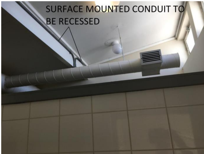
Installation to be corrected
