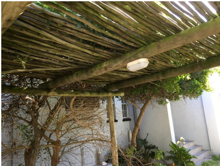
Installation to be corrected
