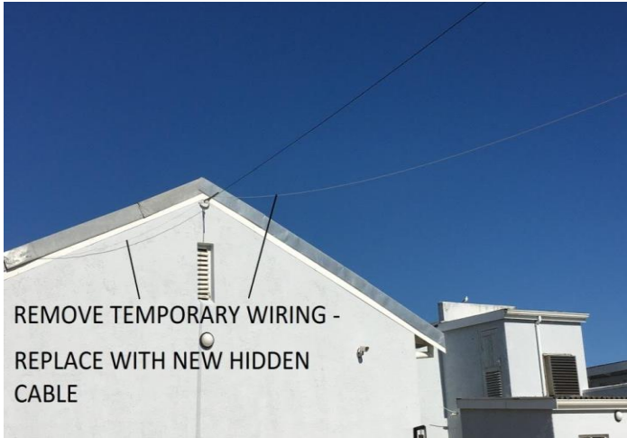
Installation to be corrected
