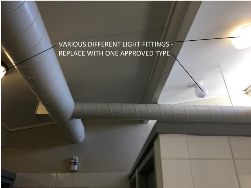
Standardise on light fittings – vapour proof type for bathrooms
