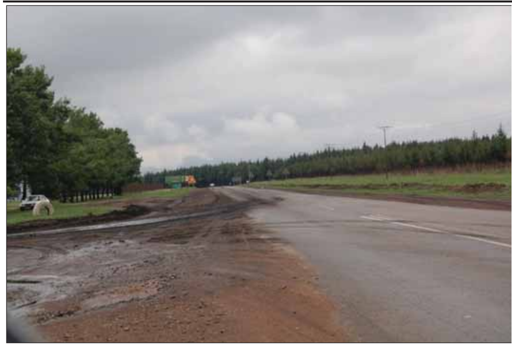
Figure 7.31 Mud Carry-over from Panbult Siding onto Public Road
