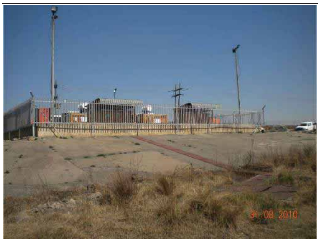
Figure 3.6 Typical Electrical Substation associated with a Main Mine Adit
