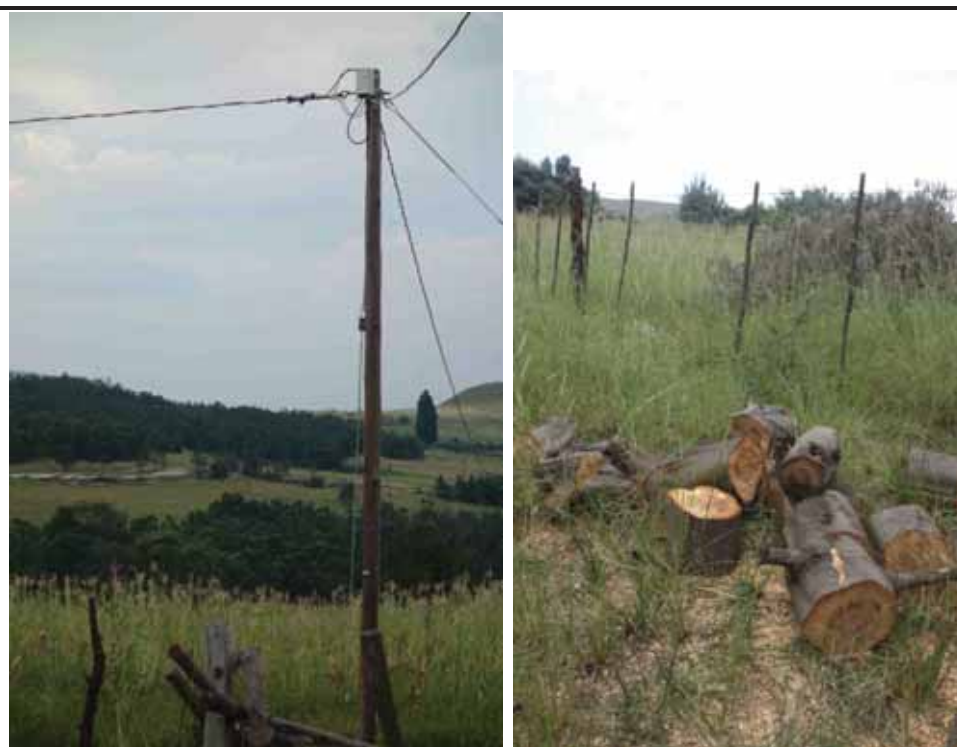
Newly installed pre-paid electricity infrastructure Firewood cut from nearby wooded area
