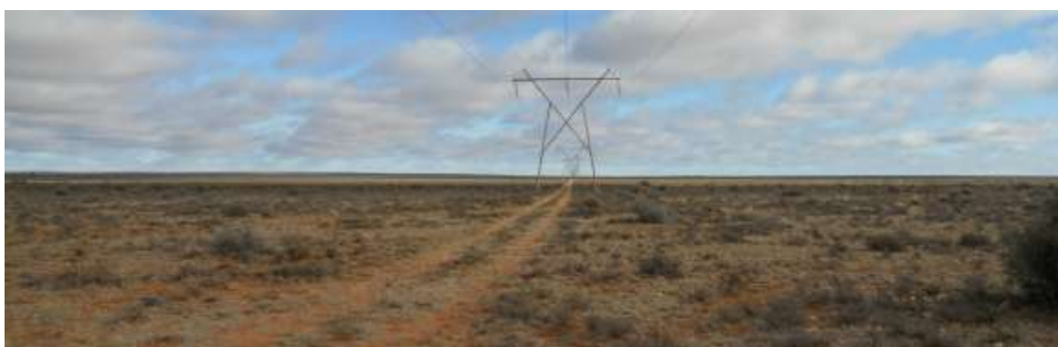
Fig 2.5. Existing 132kV lines on the site; Eskom's gravel maintenance track under the line can be seen. Source: Viridian
