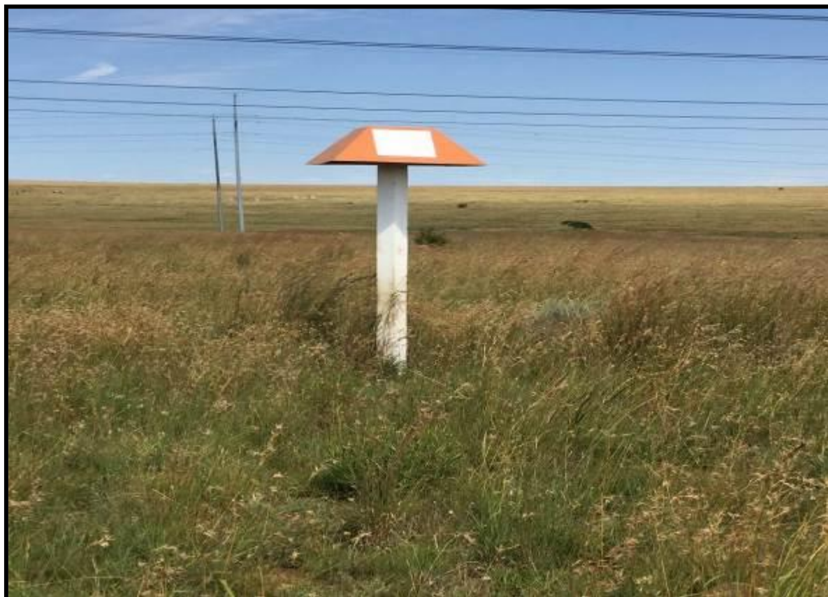
Figure 4: The existing gas pipeline within the study area (Site visit, 2018)
