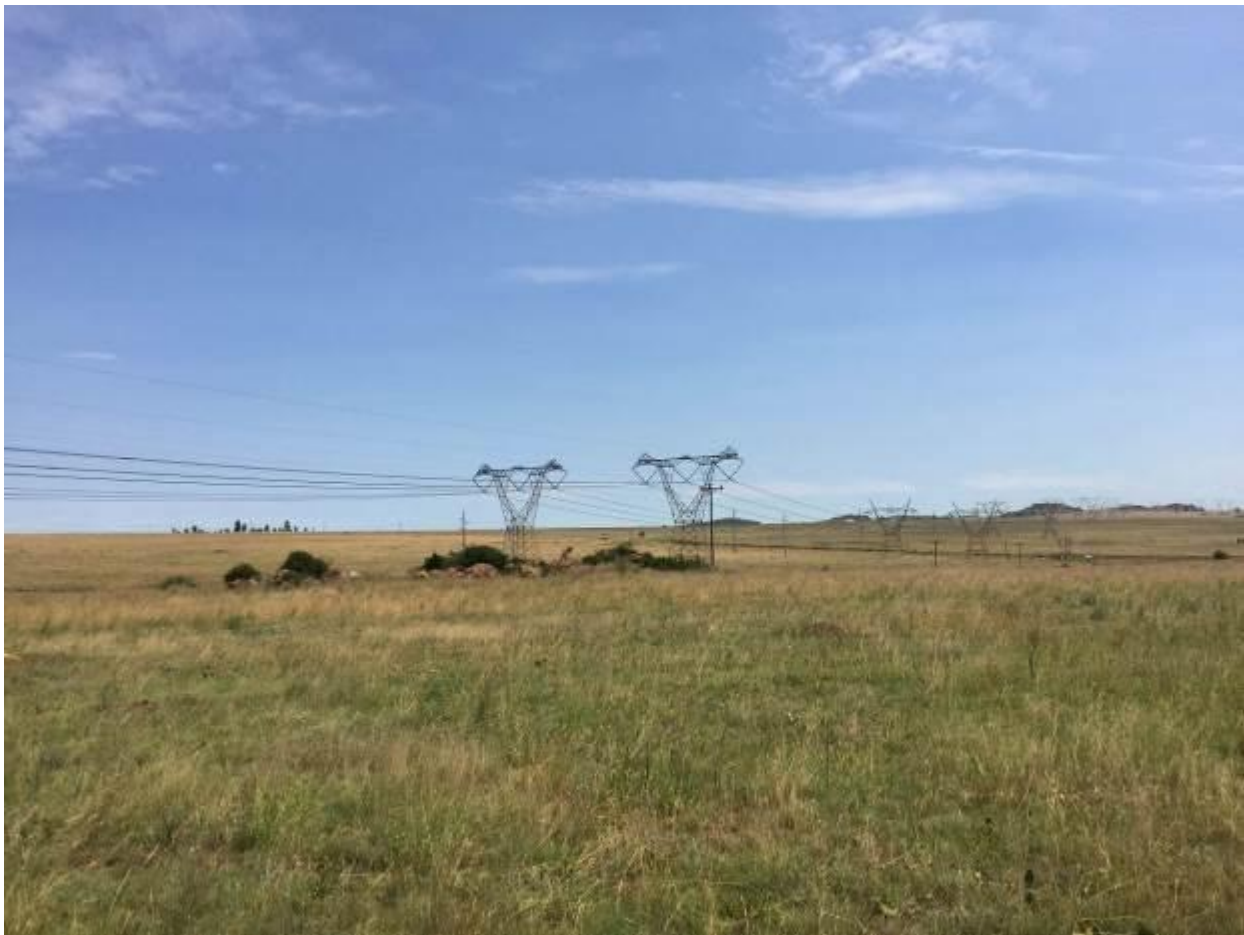
Figure 3: The existing power lines within the proposed site (Site visit, 2018)
