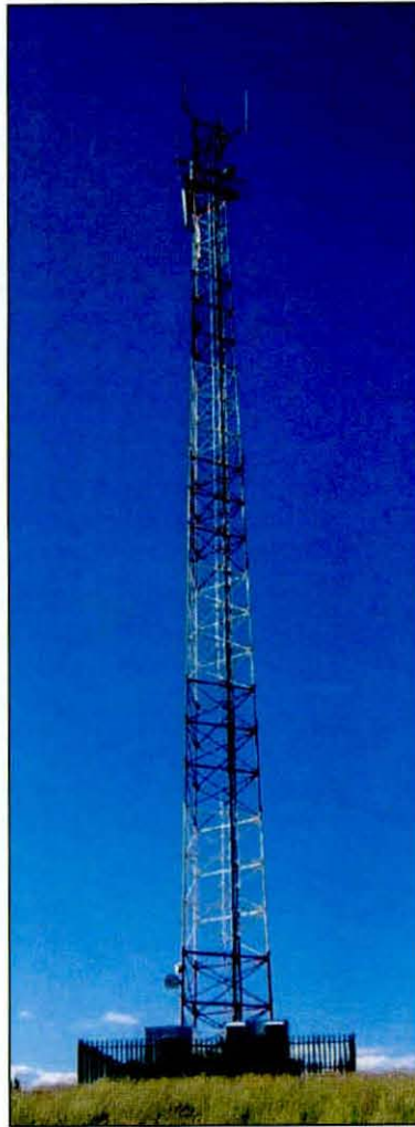
TYPICAL 3-LEGGED LATTICE MAST (PAINTED RED AND WHITE)
