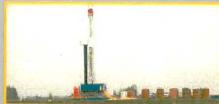
The drill site may require up to 1 ha of land. After drilling, the equipment will be removed. Land at unproductive wells will be appropriately rehabilitated.
