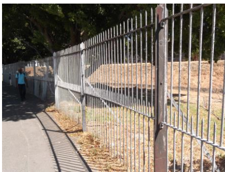
Fig 4 - Existing fence Darling Street
