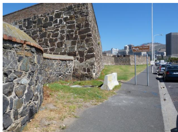
Fig 2 – Fence to end in Strand Street against the existing stone wall on the left
