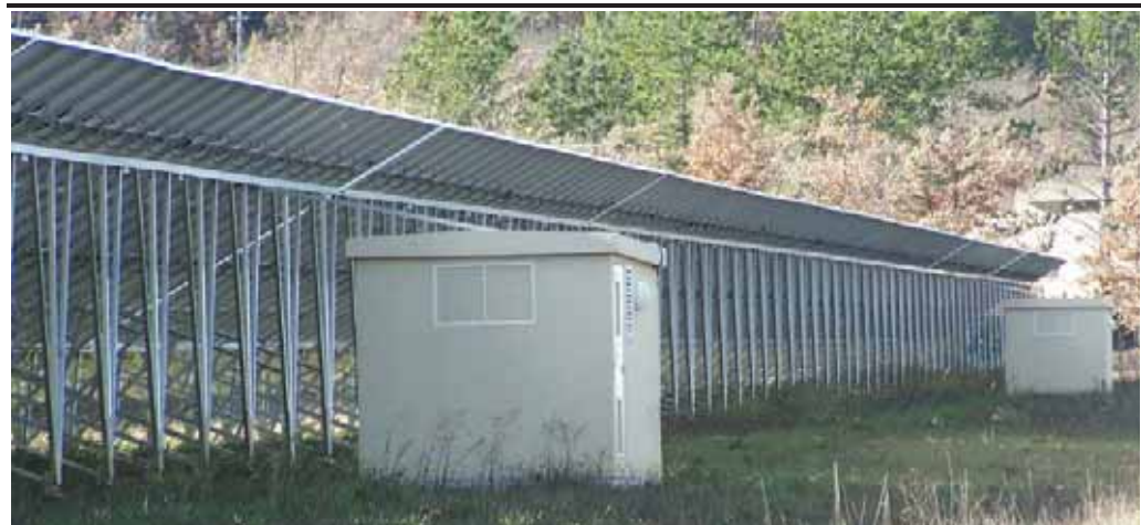
Figure 4.7 Typical Inverter/Transformer Enclosures
