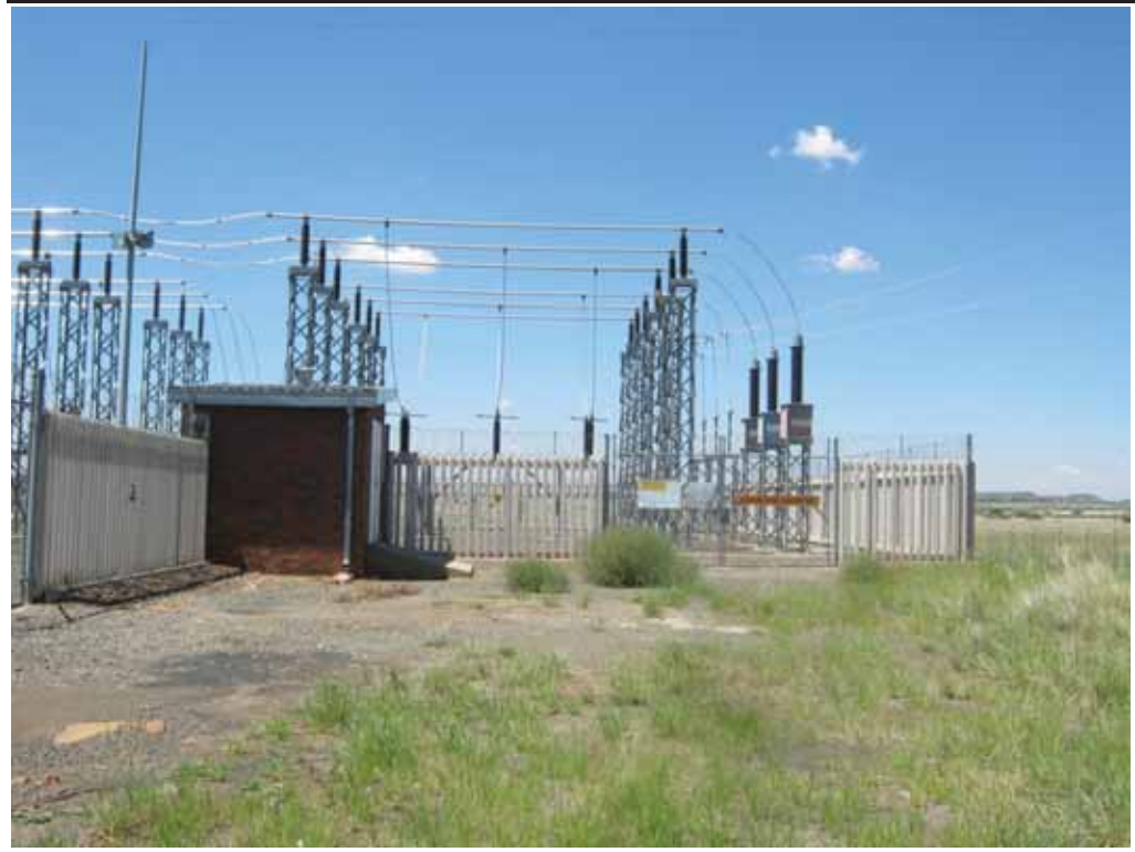
Figure 4.10 Existing Graspan Traction Substation
