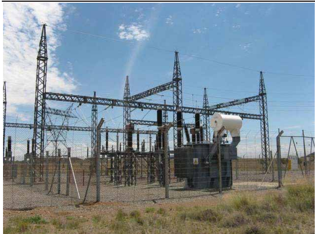
Figure 4.9 Transformer in Grid Connection Substation Yard
