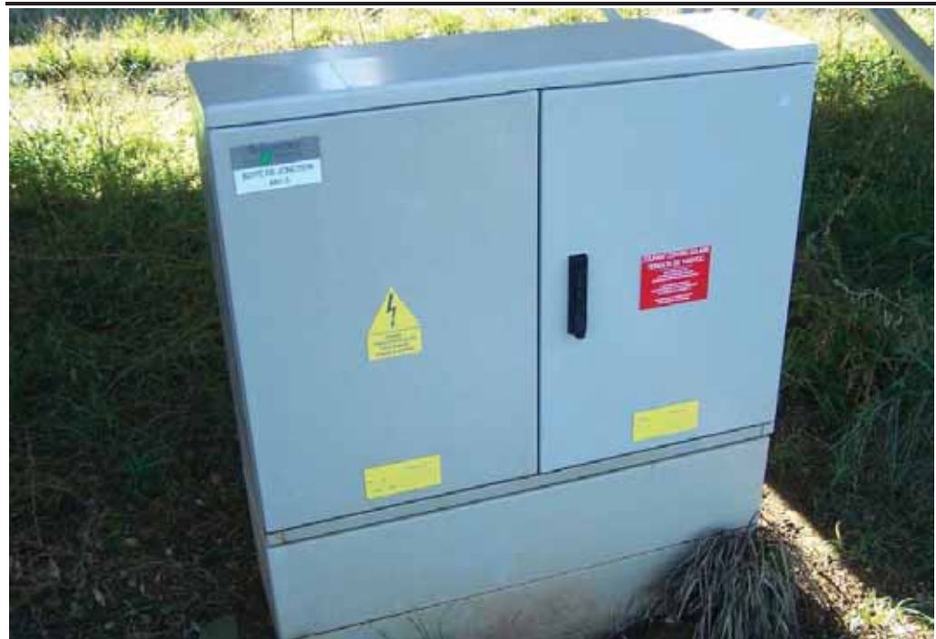
Figure 4.5 Typical Array Enclosure
