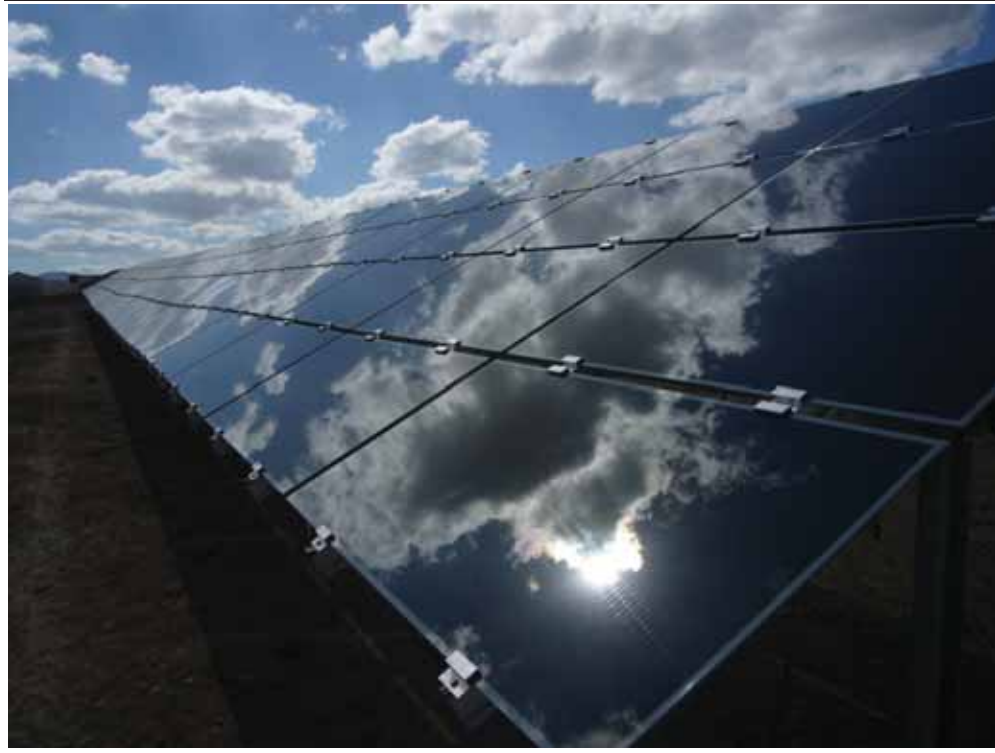
Figure 4.4 Typical PV Array
