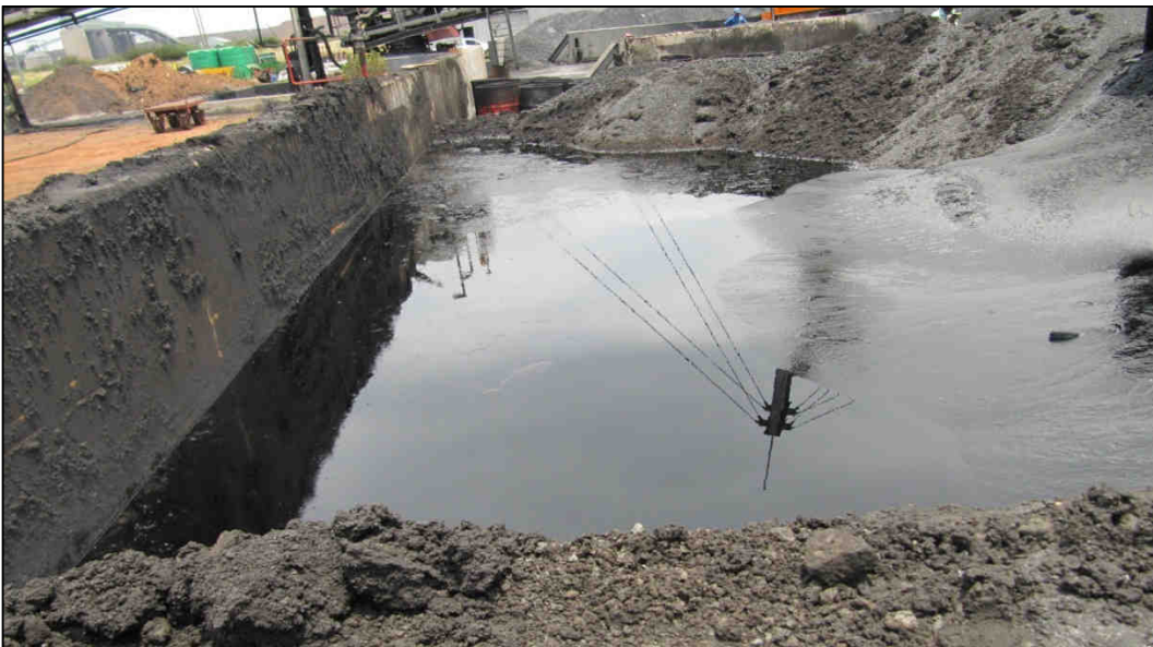
Plate 3.22: Tar sludge mixing area (currently using part of the product storage area)
