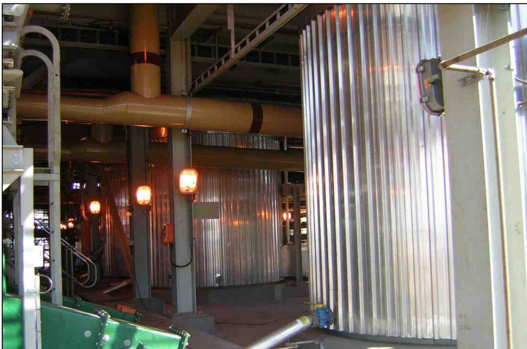
Plate 3.17: Tar storage tanks.
