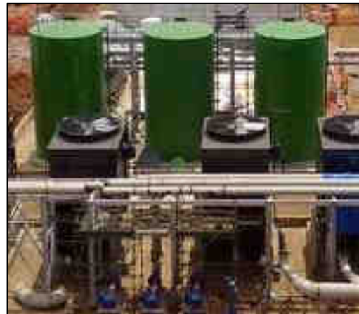
Plate 3.19: Liquor storage tanks.
