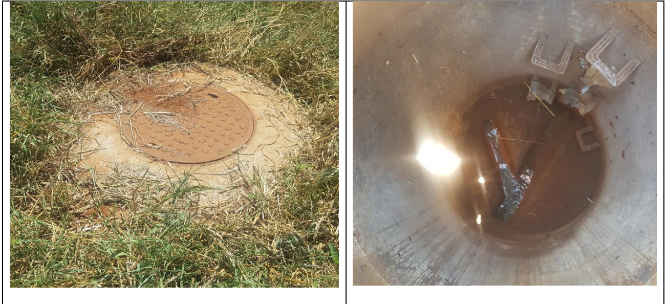
Figure 16 Sewer reticulation manhole
