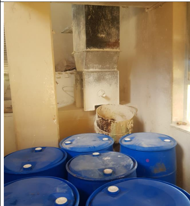
Lime machine to treat raw water is out of order and has to be induced by hand
