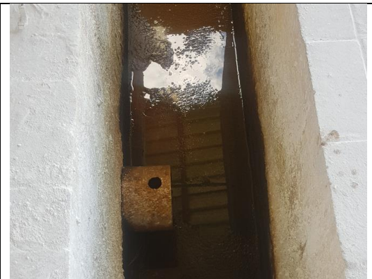
WTW inlet after treatment with coagulant and lime.
