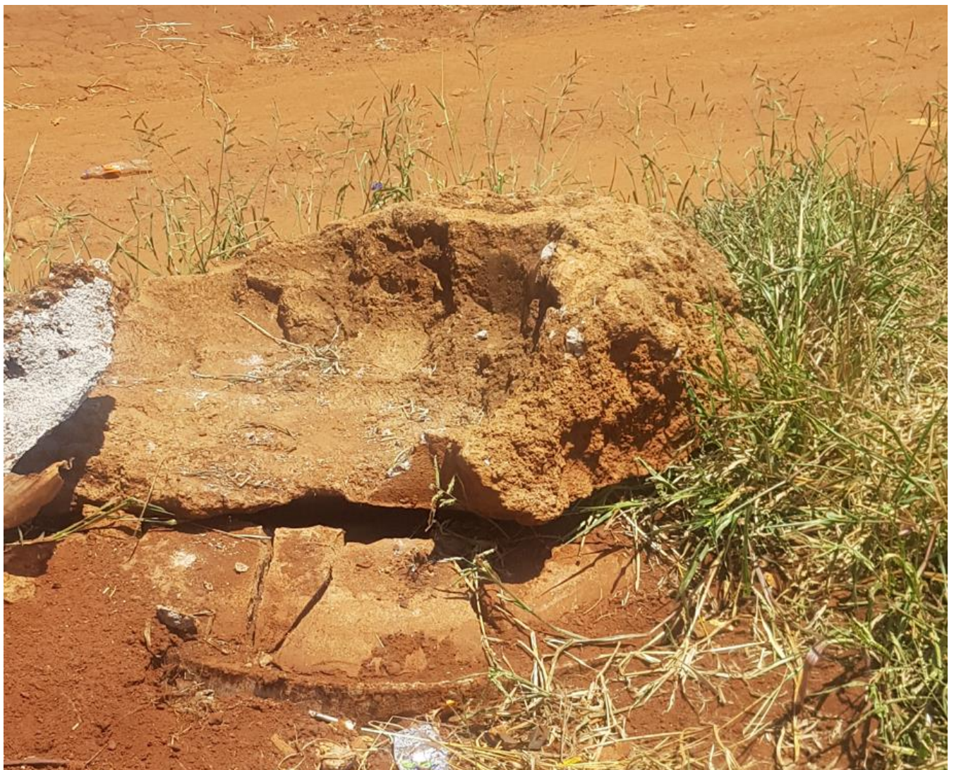
Figure 15 Sewer outfall manhole (Missing manhole cover)
