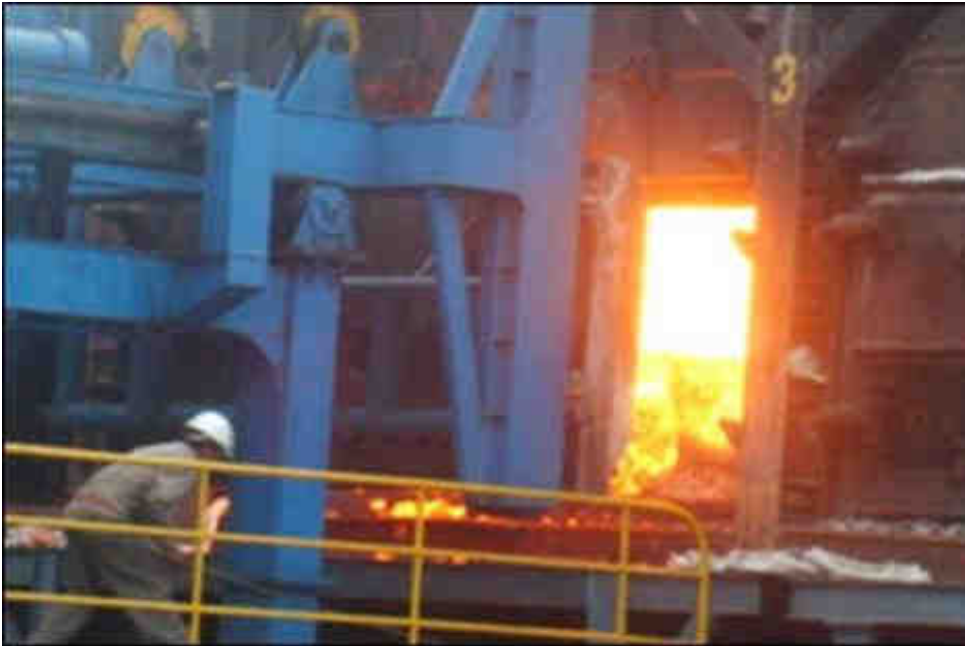
Figure 3.11: Pushing/charging machine opening coke oven door. View of heated coke cake in oven (Courtesy Sinosteel)
