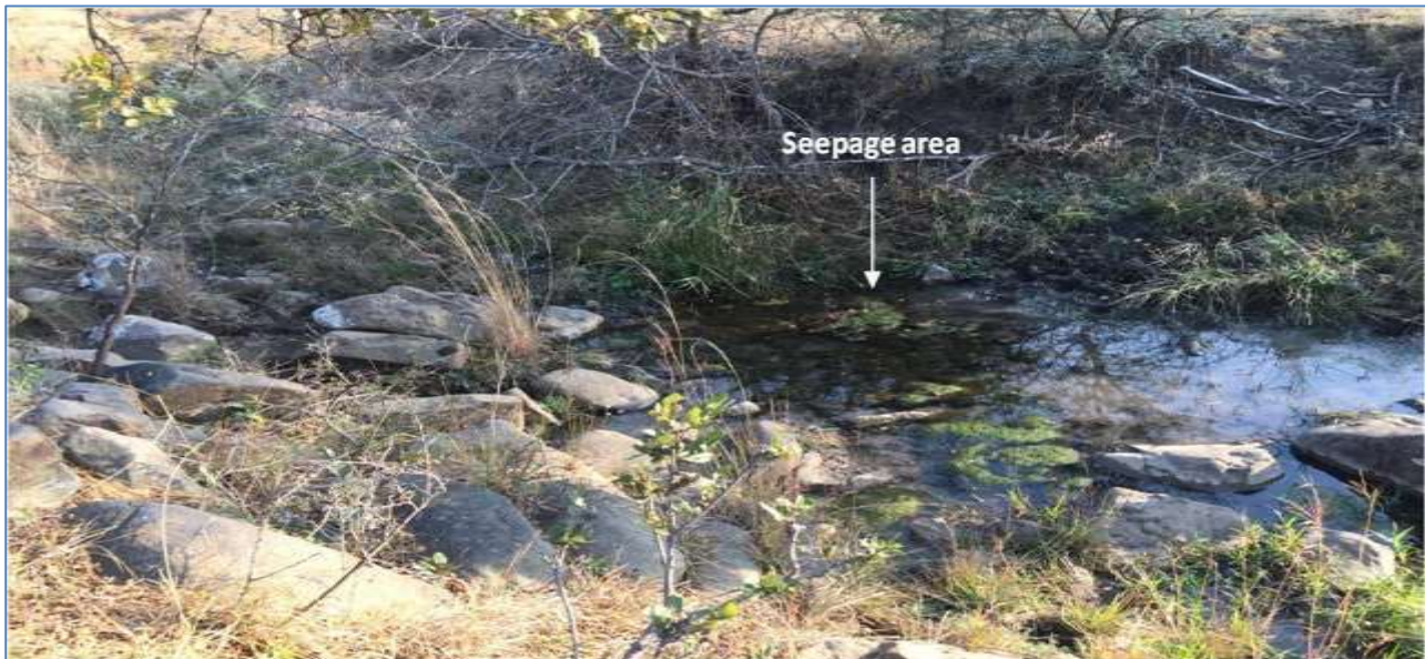
Figure 5-30: Seepage area / wetland present at the edges of the man-made dam
