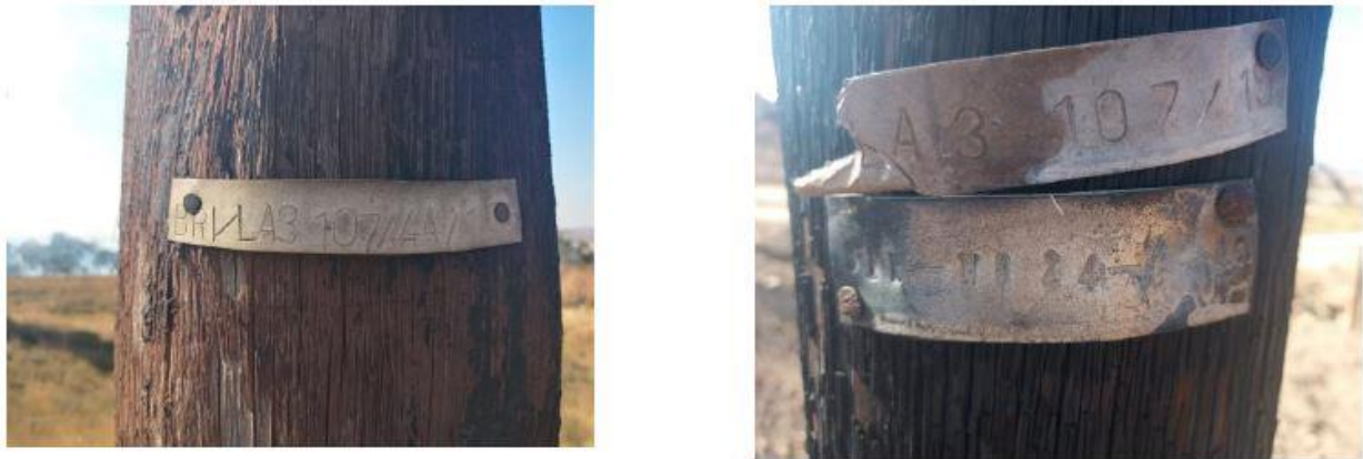
Figure 7: Eskom Pole BRI/LA3 107/4A/1
