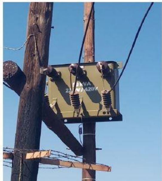
Figure 6: Eskom Pole BRI/LA3 107/13
