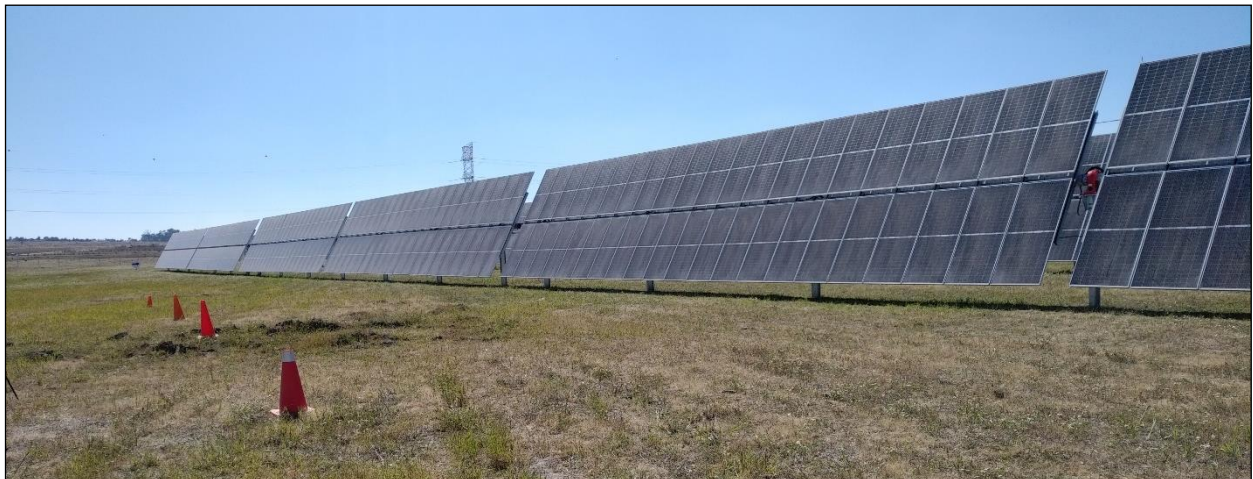
Figure 6. Frontal views of the PV arrays mounted on horizontal 1-axis tracker
