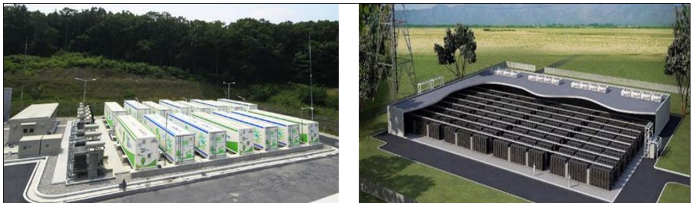
Figure 8. Battery Energy Storage System (BESS)
