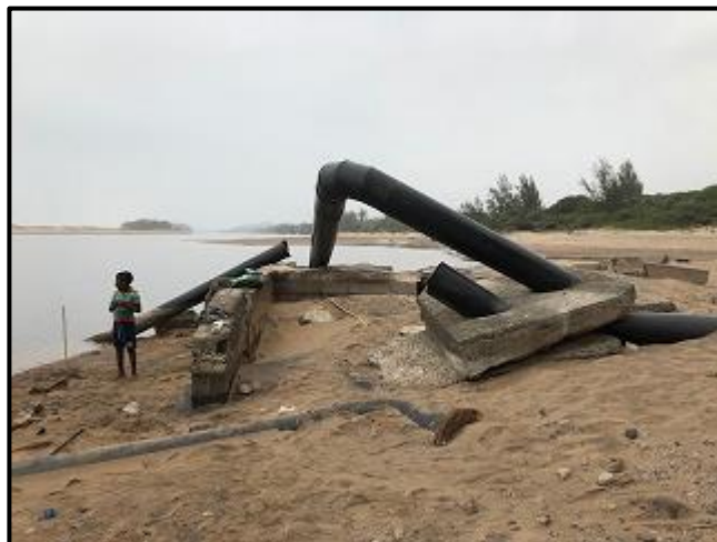
PLATE 2: PUMPHOUSE ON AMATIKULU LAGOON
