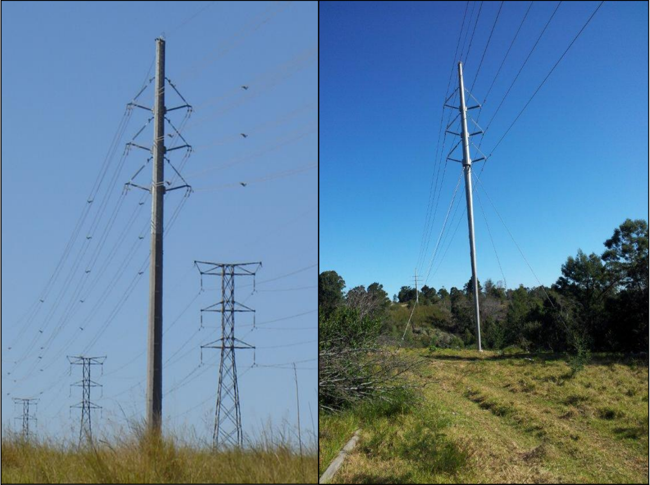
Figure 2: Examples of steel monopole structures.
