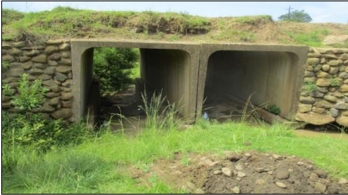
Photo 3: Showing upstream view of No. 2 cell concrete box culverts at crossing No. 3 with stone pitched wing walls.
