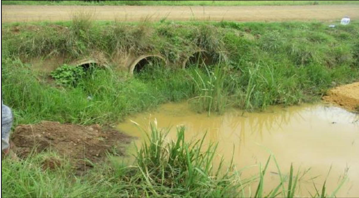
Photo 5: View of 3 No. cell concrete pipe culvert with debris accumulation and water ponding at water crossing 5
