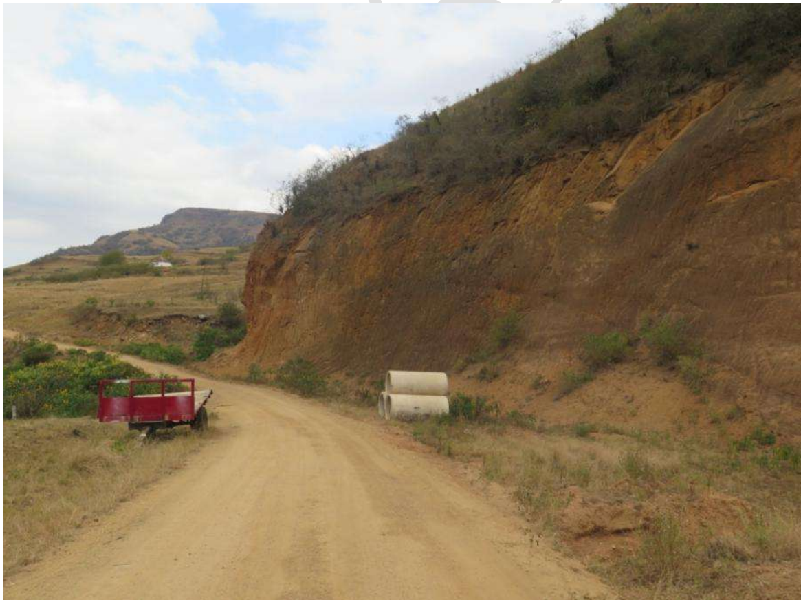
Photo 14: Quarry face directly adjacent to Mzumbe River. Top is unstable and will most likely collapse with big rain. Stream running under road and into the river in background left.
