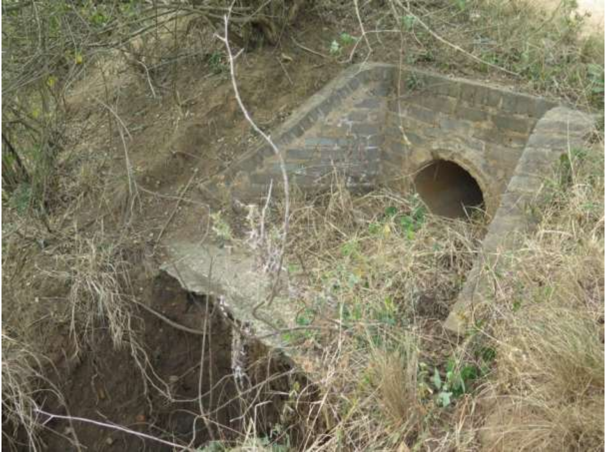
Photo 11: Outflow from drainage under the road that has not been designed to allow dispersion of water energy.
