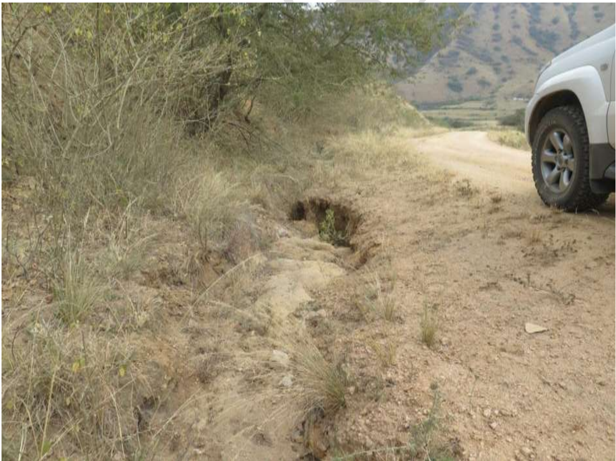
Photo 10: Erosion on D168 due to inadequate water dispersion.
