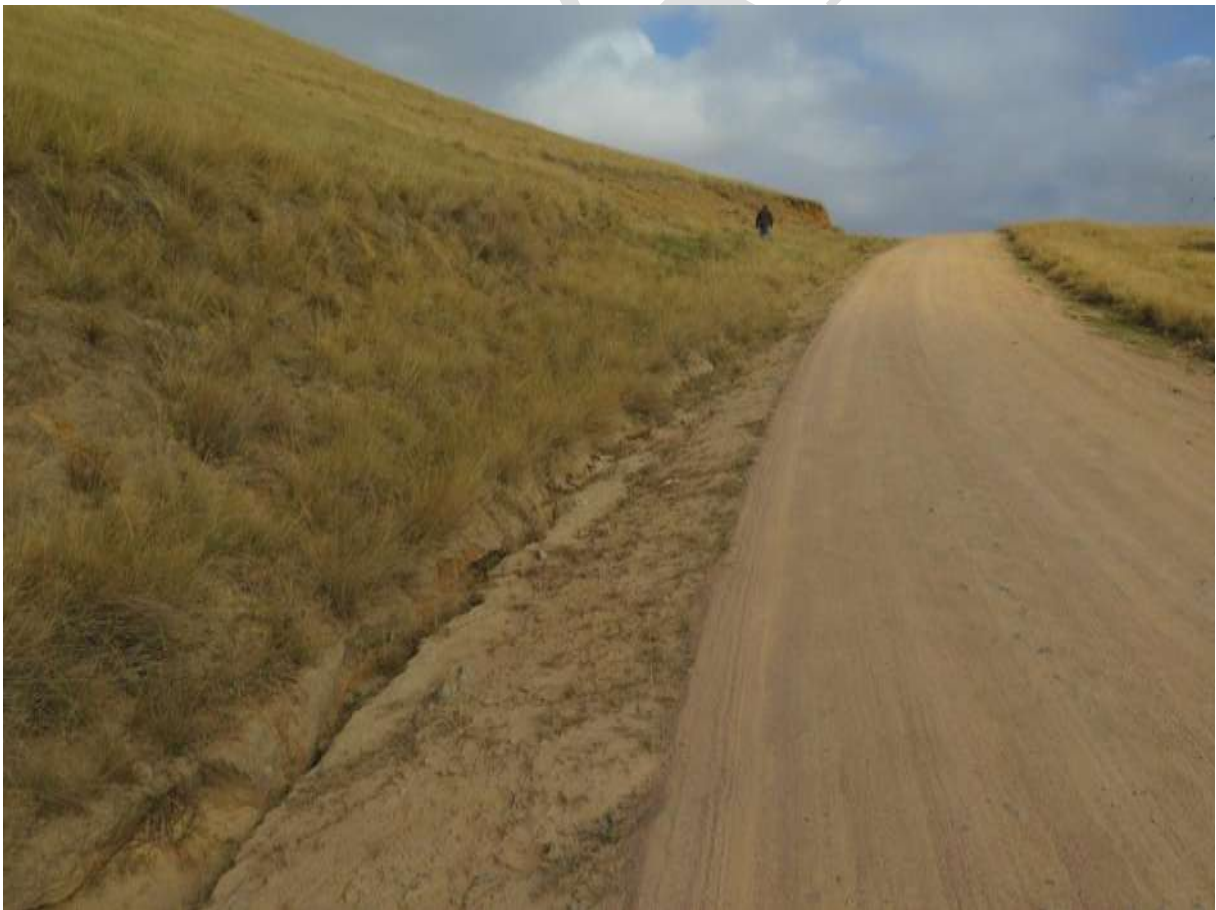
Photo 2: Example of erosion on D168 due to inadequate dispersion of water from road surface.
