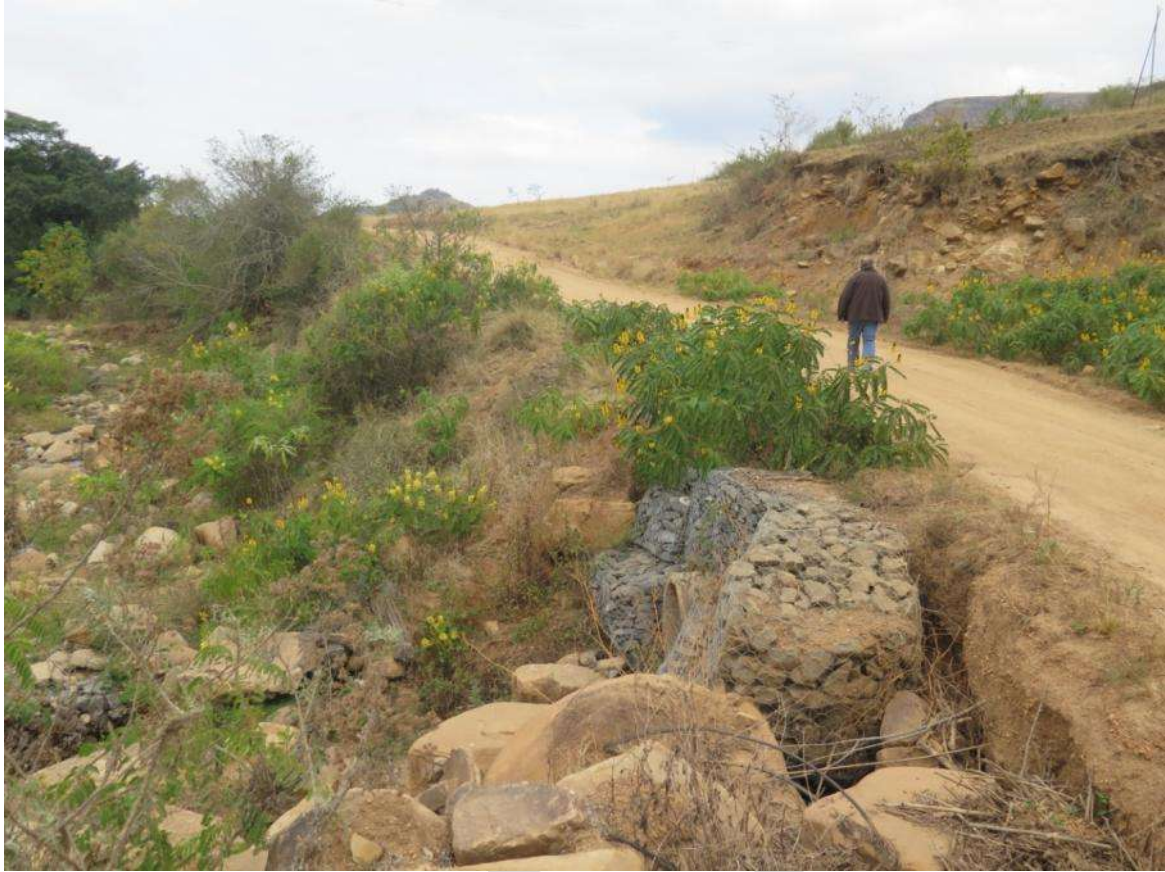
Photo 15: Stream running under D168 and into Mzambe River adjacent to quarry face shown in Photo 14. Note erosion around gabions.
