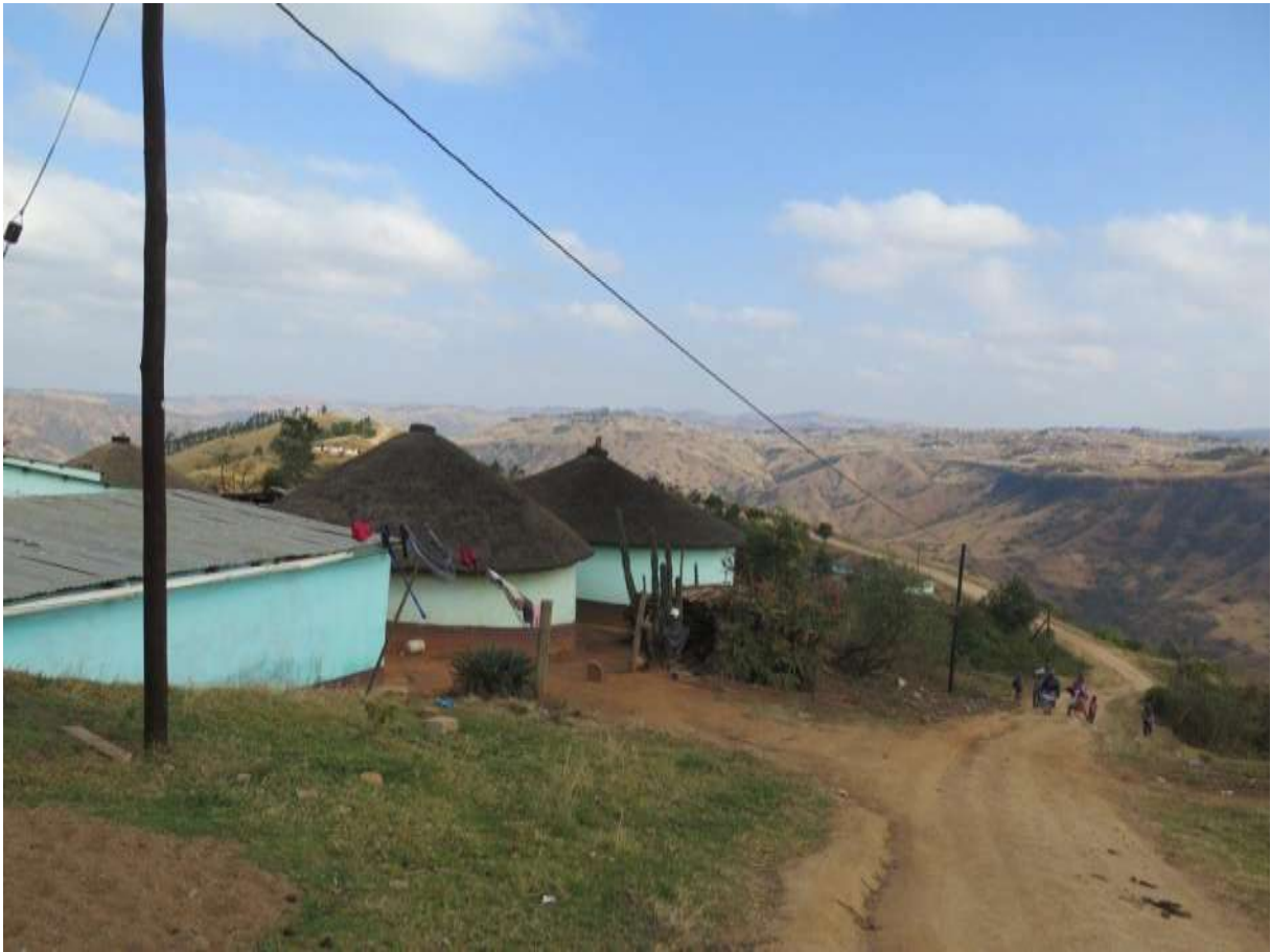
Photo 9: D167 going down steep hill past rural homesteads – drainage is a problem here.
