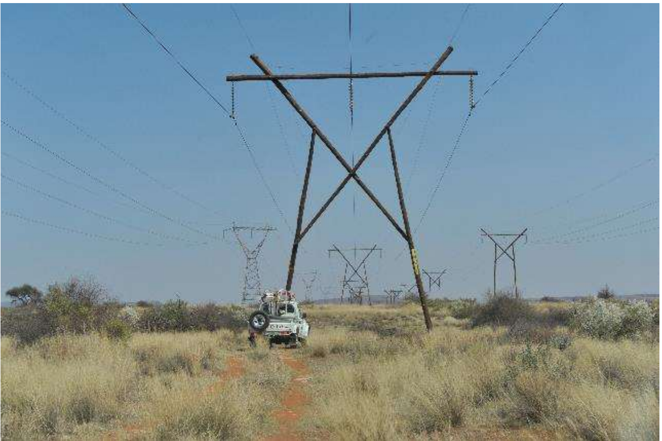
Figure 4: Existing 132kV Bulkop-Ferrum (left) and 132kV Ferrum-Sishen (middle) high voltage lines in the study area.
