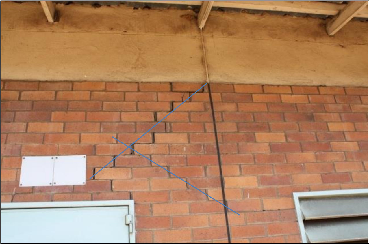
Figure 7: Example of blast induced damage.
