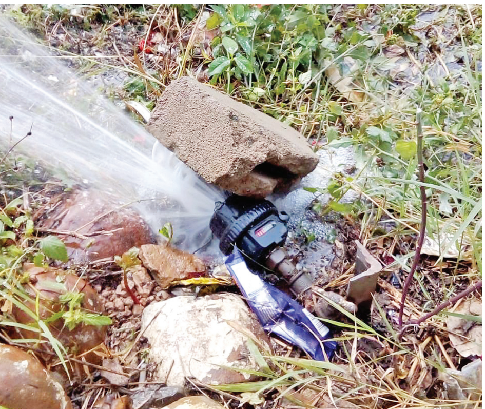
A burst water meter on Waterfern Place, Redfern, Phoenix.
