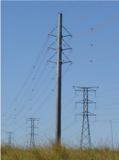
Figure 2.2: A self-supporting structure along a straight section, with a guyed angle strained structure at each bend in the alignment. Source: Aurecon
