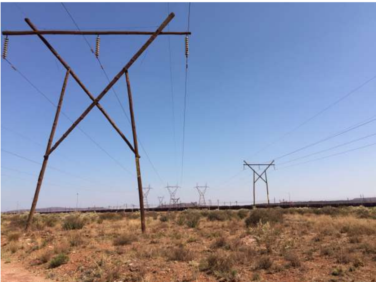
Figure 17: View south from Photo 5 of the existing 132kV Bulkop-Ferrum powerline line as well as a section of the existing Ferrum-Sishen power line which will be decommissioned and removed. The higher VAC levels of the adjacent railway line infrastructure would reduce visual contrast generated during de-construction.
