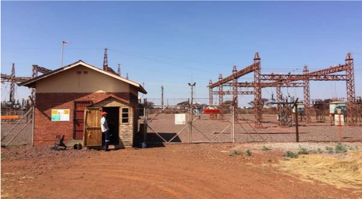
Figure 16: View from Photo 4 of the existing Lilyveld Substation
