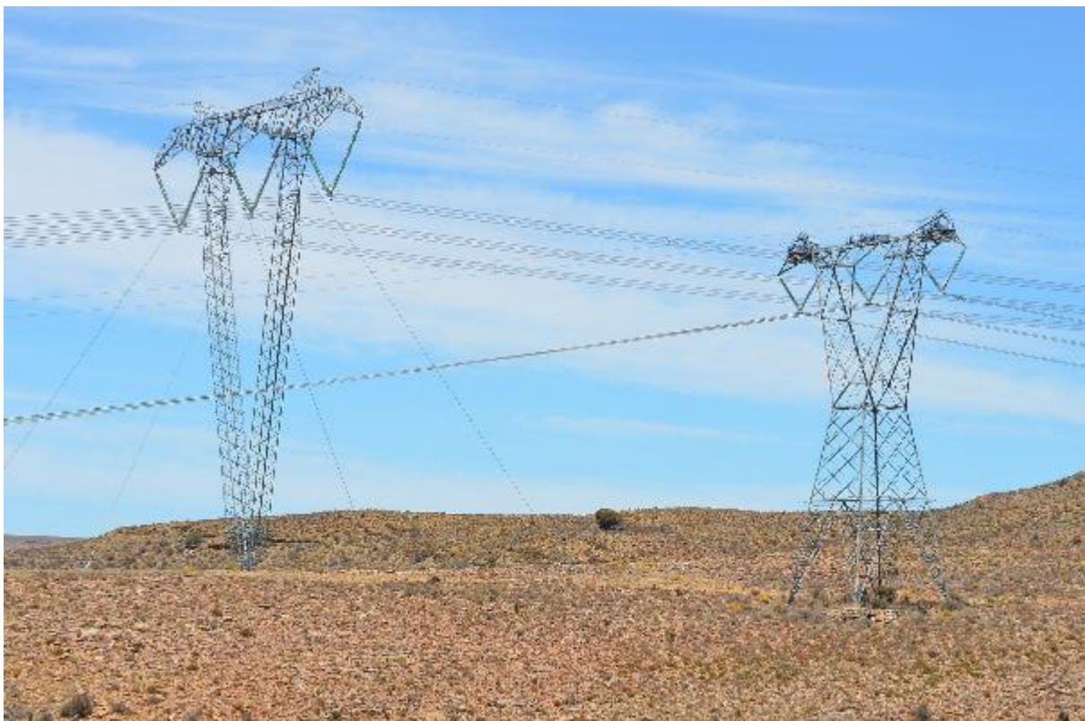
Figure 4: Existing HV lines in the study area.
