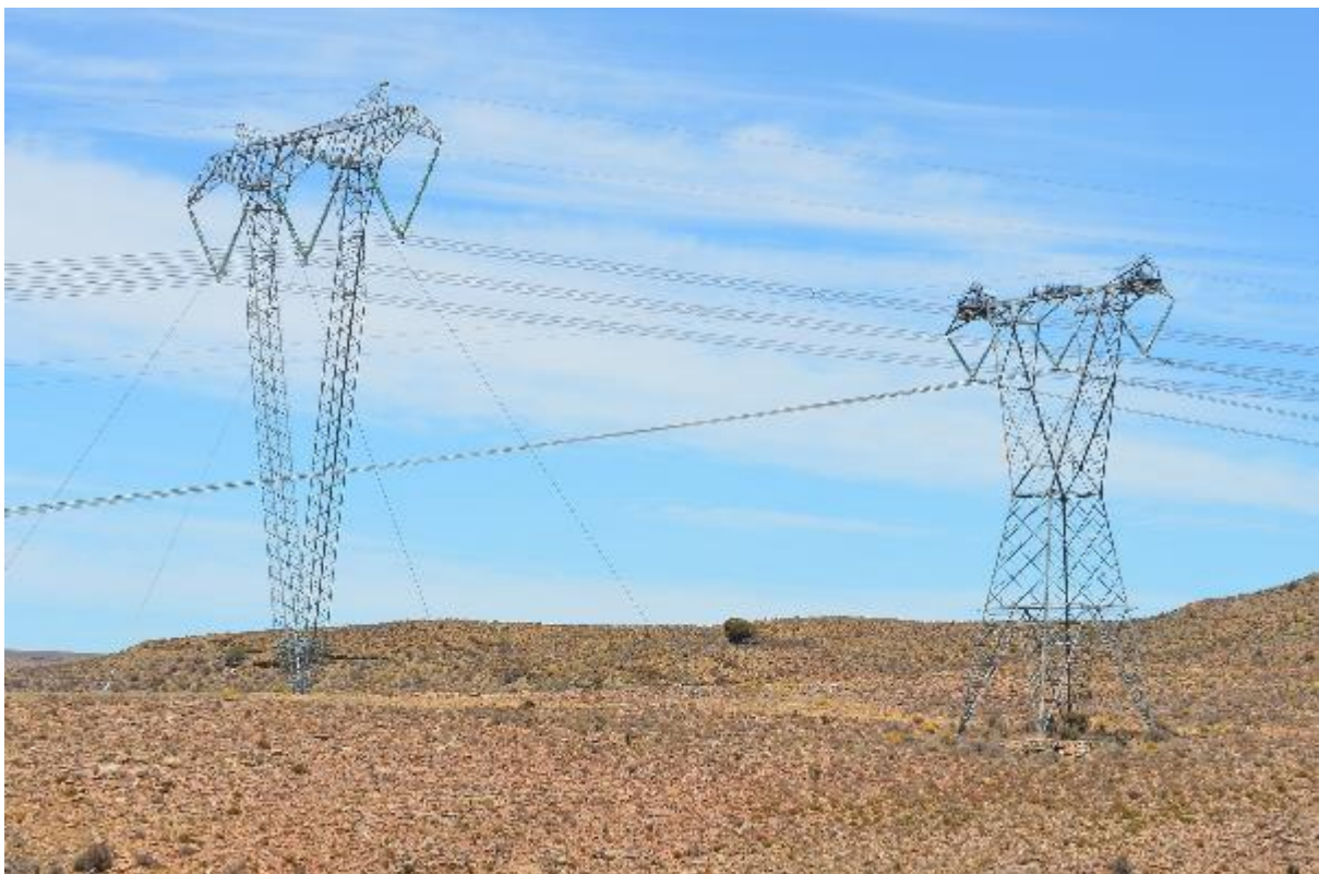
Figure 4: Existing HV lines in the study area.
