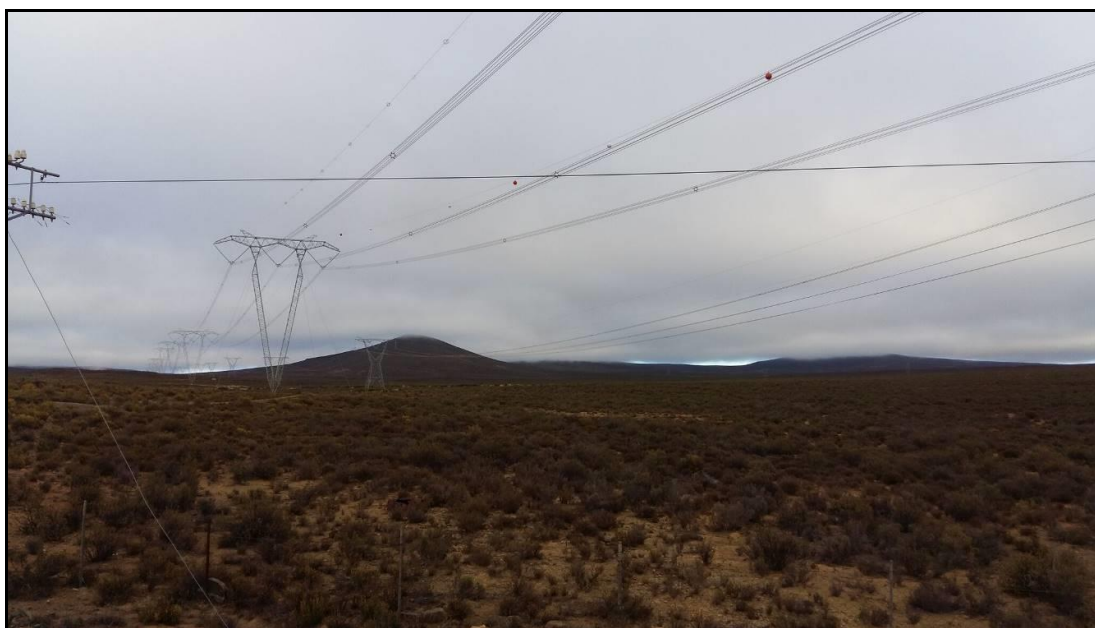
Plate 1: The landscape around the Komsberg substation, indicating the electrical infrastructure which dominates this landscape.
