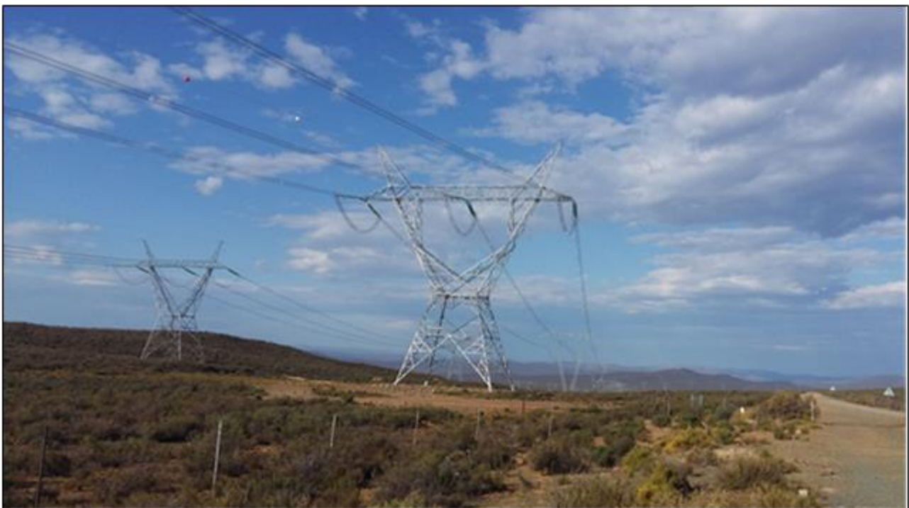
Plate 4: View of powerlines from the Komsberg substation.
