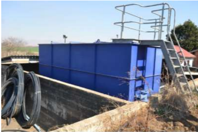
Figure 14: Existing package treatment plant
