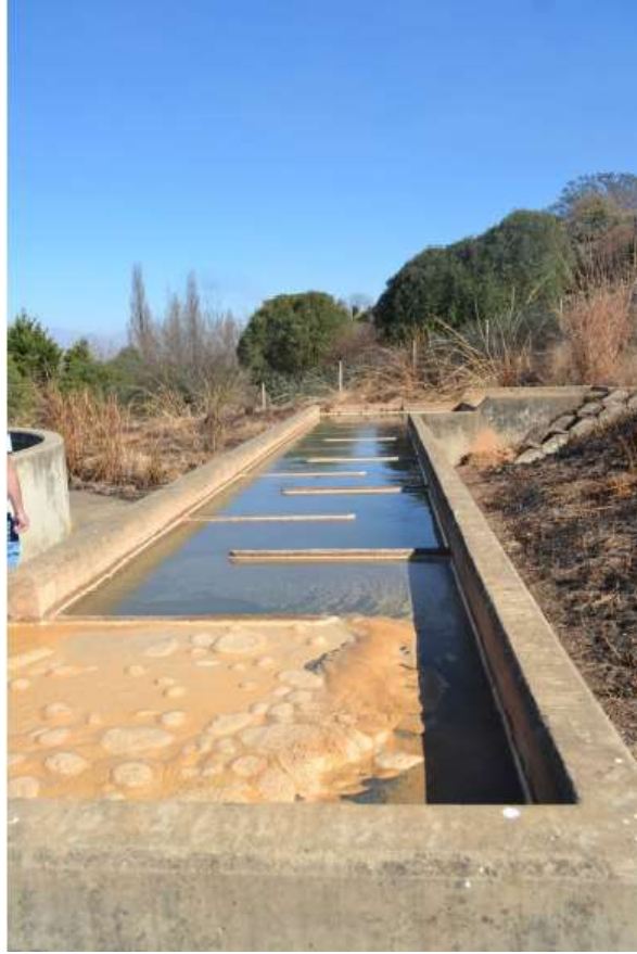
Figure 6: Lower section of flocculation channel
