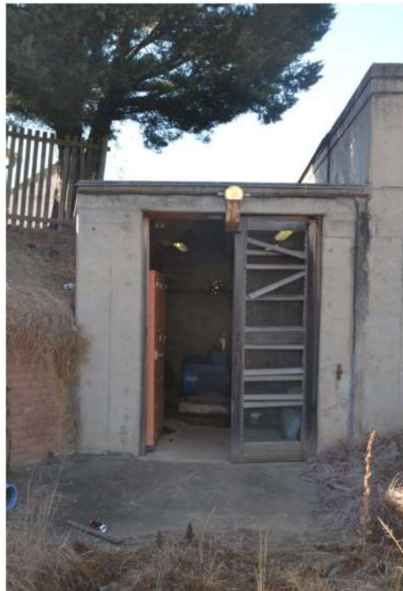
Figure 12: External view of clearwater pump station
