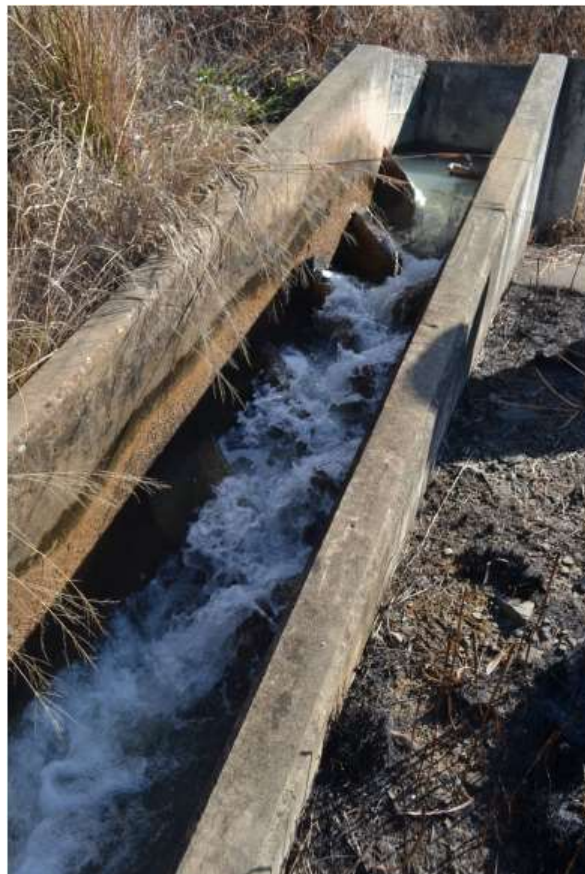
Figure 5: Upper (sloped) section of flocculation channel
