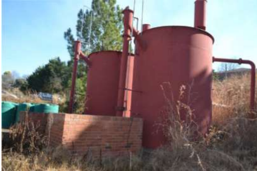
Figure 9: Auto-backwash gravity filters
