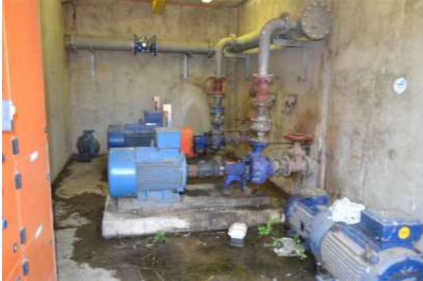
Figure 13: Clearwater pump station pumps and pipework
