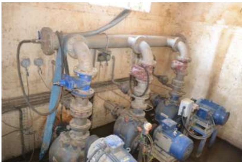
Figure 2: Raw water pump station pumps and pipework
