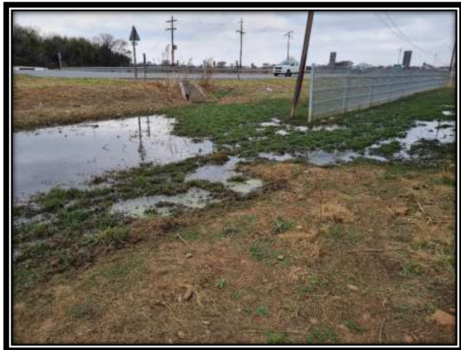
Photograph 7: Fowl-smelling water is present within the road reserve of the R503.
