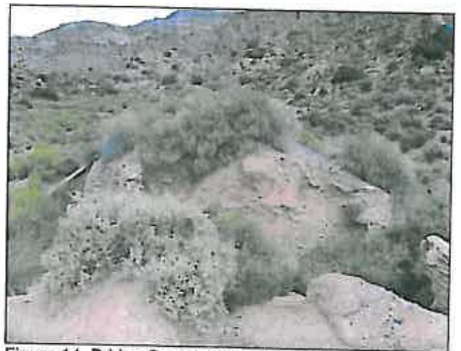
Figure 14. Bridge Crossing 1 (collapsed)
