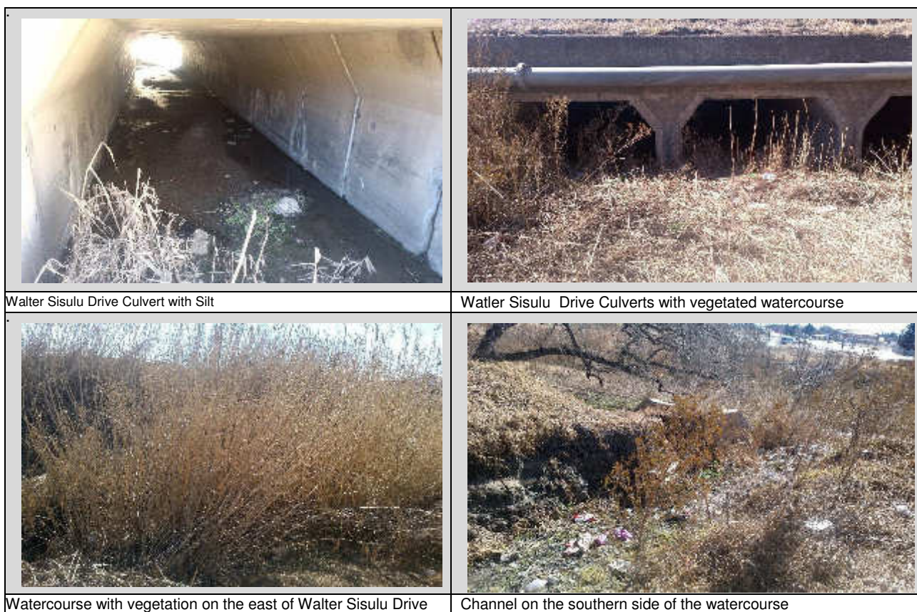
Figure 5-1: Photos taken during site visit showing the existing conditions of river and floodplains.
