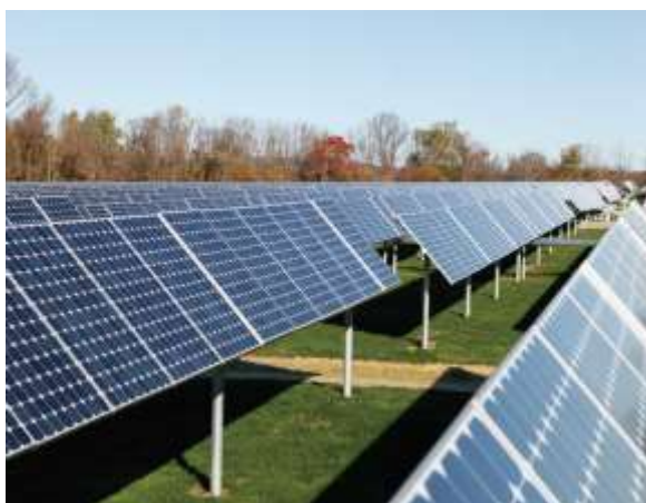
Figure 4.1.: Example of a typical single axis tracking system for solar technology
