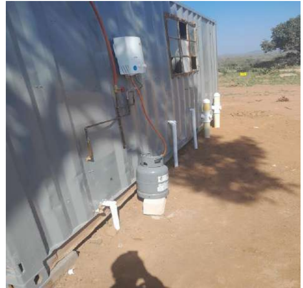
Ablution Facility with Septic Tank
