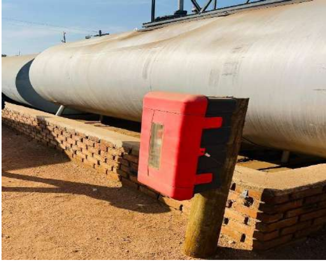
Aboveground Storage Tanks Area (500 m3)
