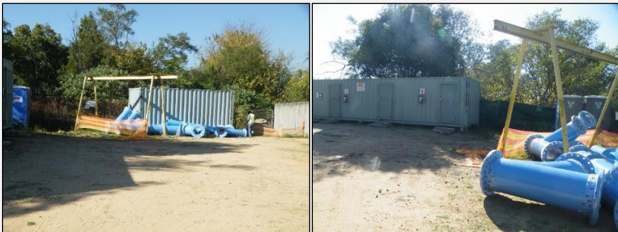
Photograph 1: Site cleared and used for construction related activities, east of existing pump station and within the proposed development footprint
