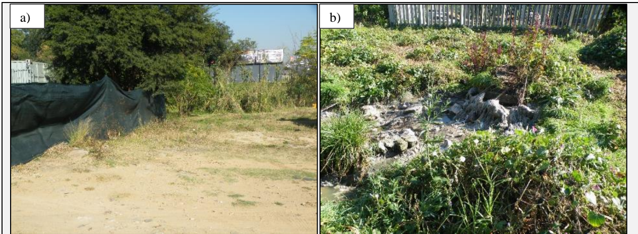
Photograph 2: a) Compacted soils at the entrance to the site and b) overflowing manhole south of the existing pump station and within the new proposed footprint
