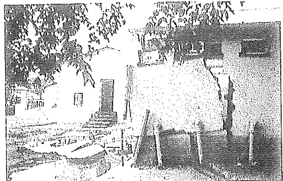
PLATE 9: BUILDING MOVEMENT AS RESULT OF DOLINE FORMATION
