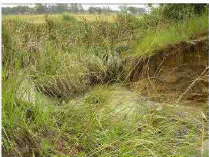
Figure 6: Downstream view of the WV2 site, indicating the significant erosion at this point.
