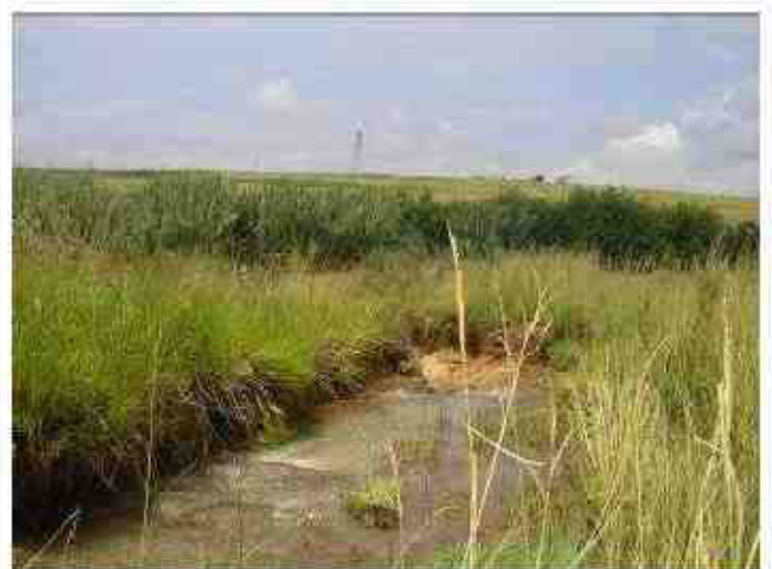
Figure 7: Upstream view of the WV2 site indicating the bank instability at this point.
