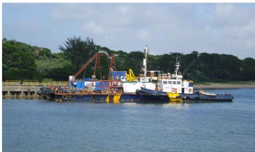
Figure 10-1: A barge and support vessels similar to what will be used for tunnelling of the marine pipelines.
