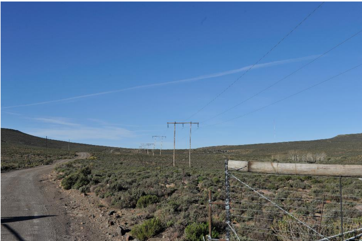
Figure 2: Existing Laingsburg / Roggeveld 1 66kV distribution power line infrastructure running north-east of the site.
