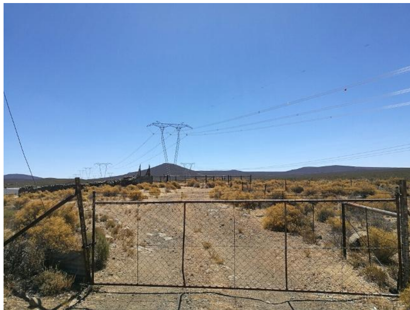
Figure 19 Power pylons near the R354
