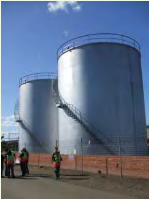
Figure 78: Fuel storage Nsezi Yard
