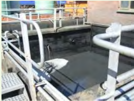
Figure 79: Separation tank at Nsezi Yard
