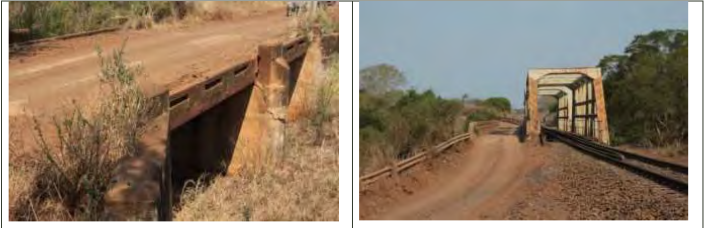
Figure 89: Concrete road bridge near the railway line and an example where they share the same substructure
