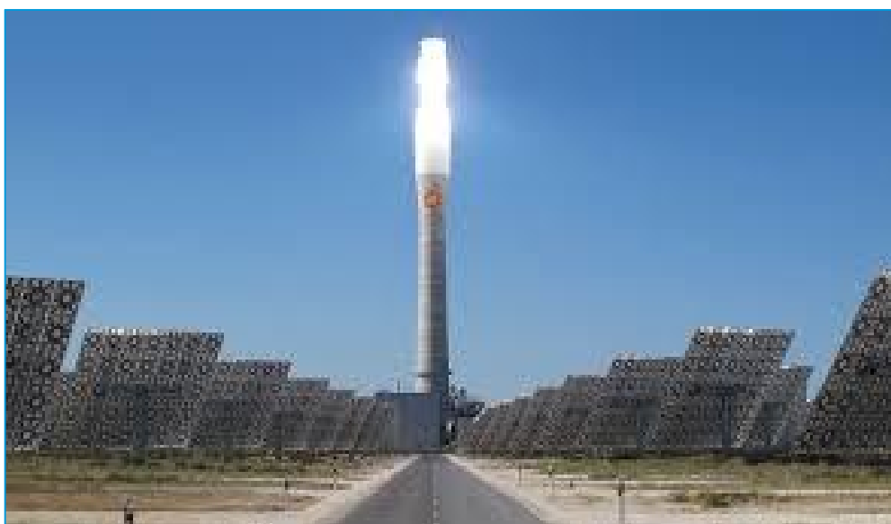
Figure 1-2: Central Tower Receiver
